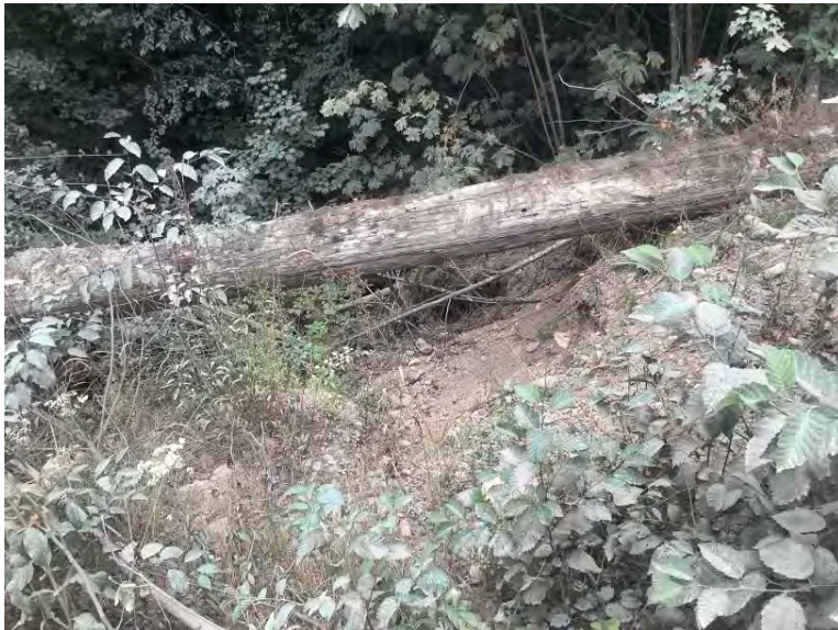
Slope failure to woods 1800
